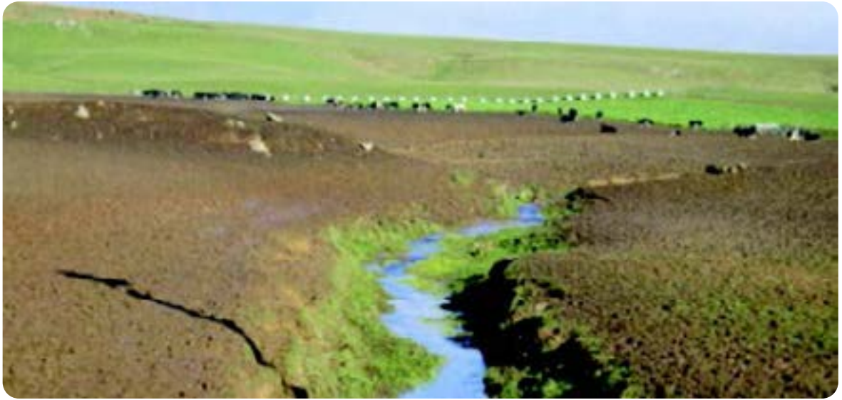
Photo 3: Post winter grazing of an unprotected gully. (Note this photo was taken before IWG regulations came into effect).
